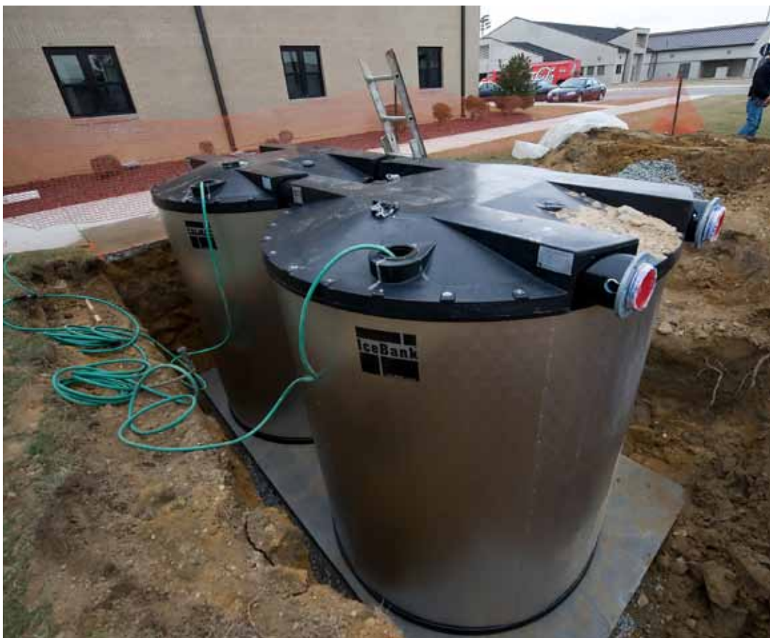
Ice storage tanks were installed at several locations on Dover Air Force Base. The tanks are part of a thermal energy storage system which will help reduce energy costs by $300,000 a year. (U.S. Air Force photo/Brianne Zimny)
