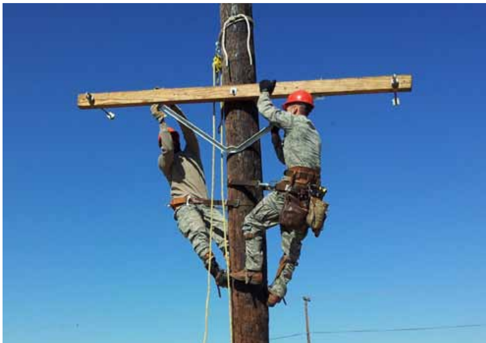
City Light and Power and Civil Engineer linemen increase the gap between each phase of the 12,000 volt primary lines at the Travis Air Force Base Duck Pond. This project aims to reduce nuisance power outages caused by large birds. (Courtesy photo)
