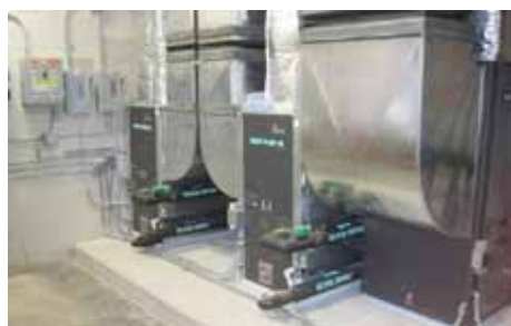
(Below) Two geothermal HVAC units are shown inside the 23rd Space Operations civil engineer warehouse facility. Engineers expect to save $40,000 in utility costs this year thanks to the installation of three systems at New Boston Air Force Station, N.H. (U.S. Air Force photo)
