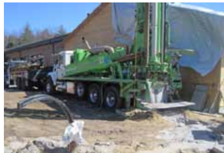
(Above) A machine drills one of 15 geothermal system wells outside the 23rd Space Operations Squadron civil engineering warehouse. Construction crews completed installation of the largest geothermal HVAC system installed at New Boston Air Force Station, N.H. in December, 2011. (U.S. Air Force photo)
