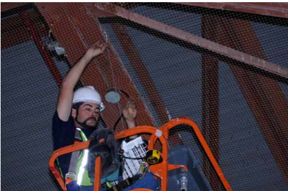
Mr. Toby Burns, a contractor, hangs new high-bay lighting in Hangar 41 at Randolph Air Force Base, Texas. The new lighting is more energy efficient and lasts longer than the existing Hangar 41 lighting. (U.S. Air Force Photo by Mr. Don Lindsey)
