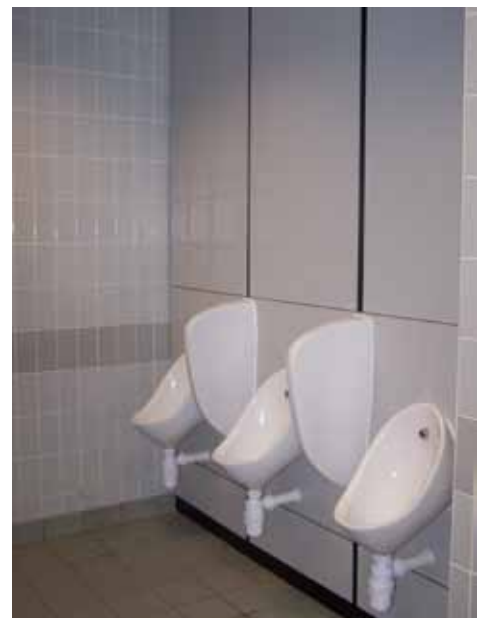
By reducing the automatic flush system for urinals at RAF Mildenhall to twice an hour during normal base work hours and once a day during weekends and non-occupancy days, water usage was reduced by 80 percent. (photo by Mr. Steve Perry)
