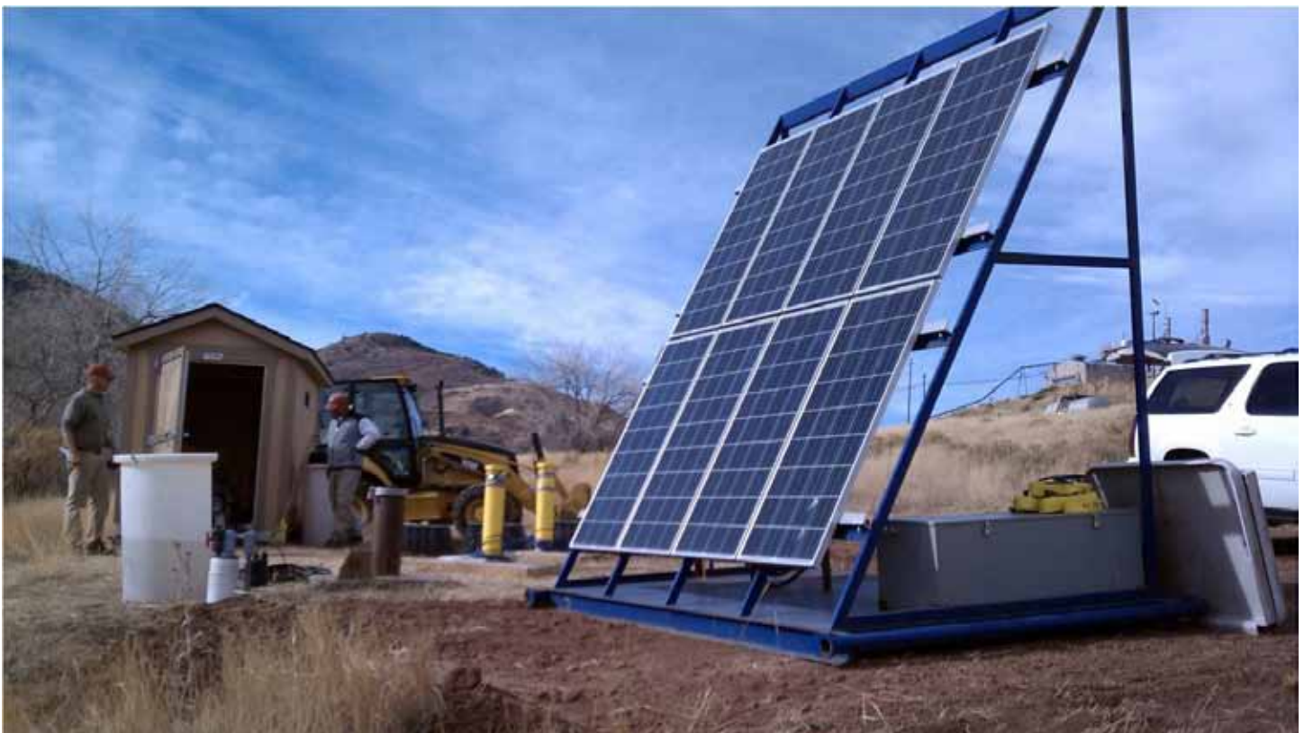
A rentable solar power skid unit - 960 watt photovoltaic array (eight 120 watt fixed mount panels) is shown here at the Air Force Plant PJKS, Systems and Components Area, in Colorado. The solar unit is powering a recirculation system treating ground water contamination. (Photo by Dr. Paul Jurena)
