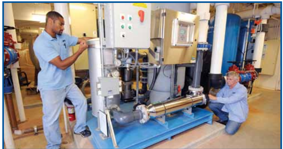
Phillip Starks, maintenance technician, left, and George Morgan, maintenance site manager of the new 72nd Medical Group facility, inspect a rain water collection system that filters and pumps the water to holding tanks where the water can be used through the facility for restrooms and in the cooling tower. Unseen by most, this system saves money, energy and ensures a non-potable water system in case of a power outage. This is one of many energy savers in systems and personnel actions that earned them a federal award for their reduced energy consumption accomplishments. (U.S. Air Force photo/Ms. Margo Wright)
