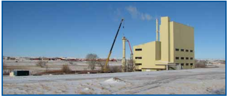
The centralized heat plant at F.E. Warren Air Force Base is scheduled for demolition as part of a $15.5 million project on base. Individual energy-efficient boilers are being installed in over 80 buildings at an annual energy cost savings of $1.6 million. (U.S. Air Force photo)
