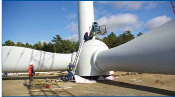
A wind project at Cape Cod Air Force Station, Mass., is moving forward watchfully as endangered eastern box turtles nest in the area. The construction area has to be swept by qualified turtle biologists, posing some slow-down to contractors, but engineers predict the project will remain on schedule. (U.S. Air Force photo)
