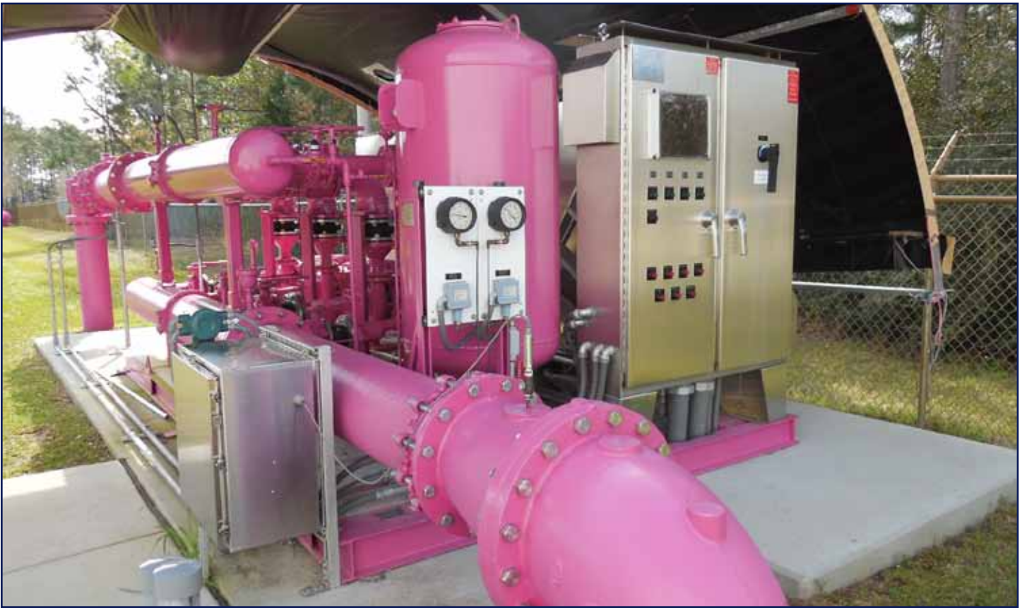
Engineers at Hurlburt Field, Fla., expanded and improved the installation's graywater distribution system to reduce demand on the local water supply. Forty-thousand feet of new piping and a 500,000 gallon storage tank help the base save 13 million gallons of potable water a year formerly used for industrial and irrigation needs. The Department of Energy chose it as a 2014 Federal Energy Management Program award winner. (U.S. Air Force photo/Released)
