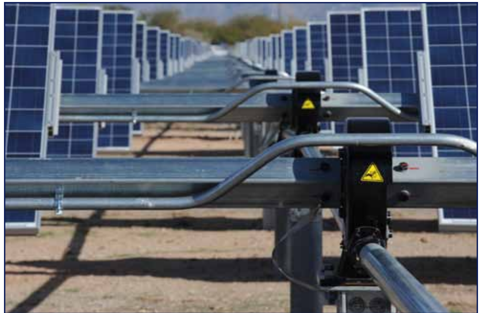
Solar panels collect sunlight at Davis-Monthan Air Force Base, Ariz. The Davis-Monthan solar array project is placed on 170 acres of underutilized land, making it the largest of its kind currently on any U.S. Department of Defense installation. The Department of Energy chose it as a 2014 Federal Energy Management Program award winner. (U.S. Air Force photo/Released)
