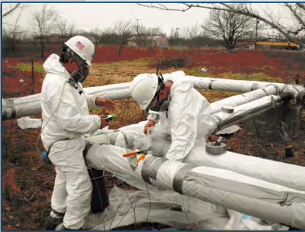
Field workers take precautions to safely prepare asbestos-insulated pipes for removal and disposal. Approximately 6,000 linear feet of piping was removed from the 900 Area of the former Chanute AFB.
