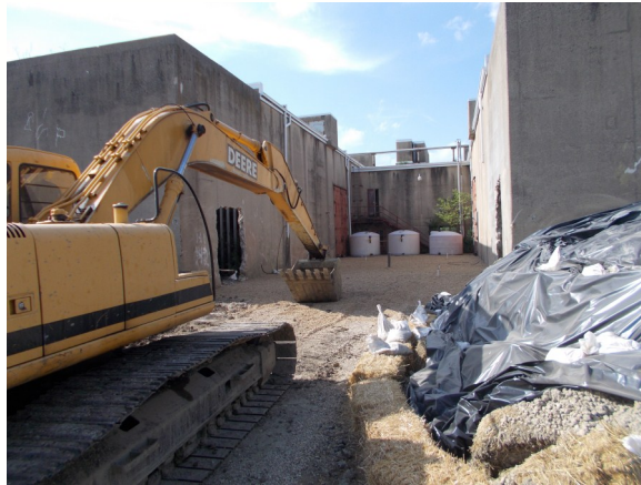
Air Force Contractor, CB&I, completes backfill of the excavation at Site SS041. U.S. Air Force Photo/Jeff Stringer/released
