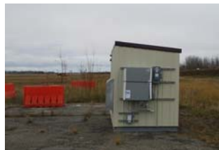
SVE blower shed at Site SS015
