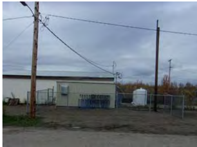
Blower Shed with Stack on Right
