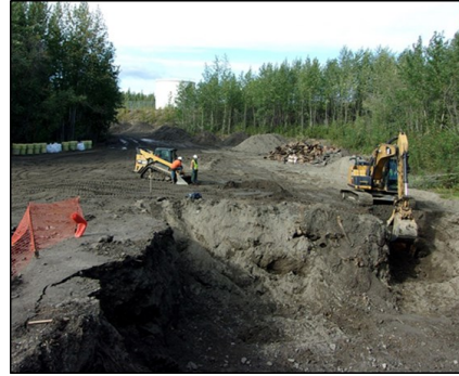
Air Force contractors excavate Site DP023. Contractors removed 6,500 yards of contaminated soil and debris from this site.
