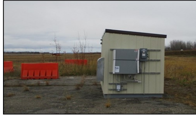
Blower shed for a soil vapor extraction system at Site SS015. Vent wells were installed at the site and connected to the blower
