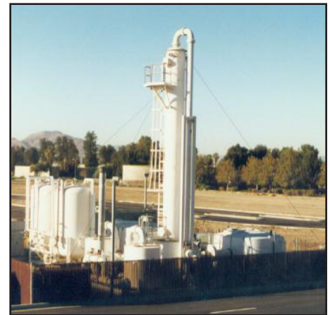
This pump and treat system was used at the former Norton AFB, Calif.
