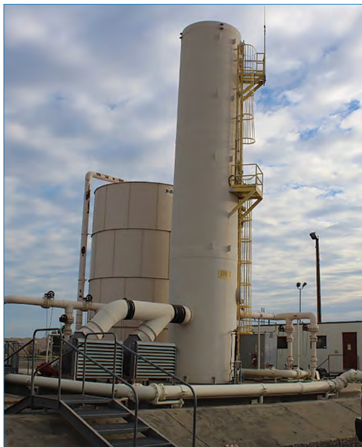
Air Force Groundwater Treatment Plant will be relocated north of its present site in 2023. Relocation will enable access to clean up contaminated soils beneath the area, and the relocated plant will operate more efficiently with new equipment and technology.
