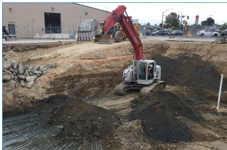
Excavation of fuel contaminated soil at site CS T-020, a former underground storage tank farm undergoes remediation. 287 privatized cleanup sites have been completed out of 296. The remaining 9 cleanup sites are now funded with work resuming in the 2022 field season.
