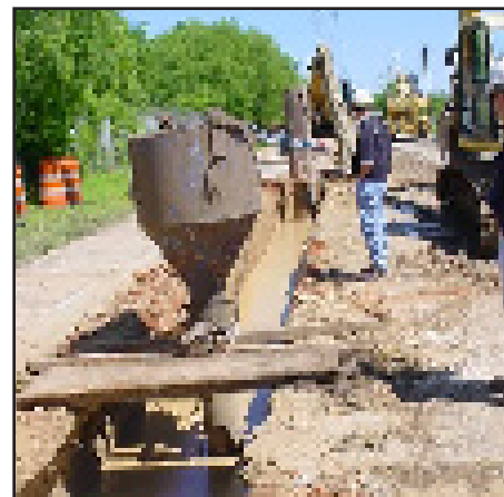
Air Force contractors install a Permeable Reactive Barrier outside the former Kelly AFB, San Antonio, Texas.
