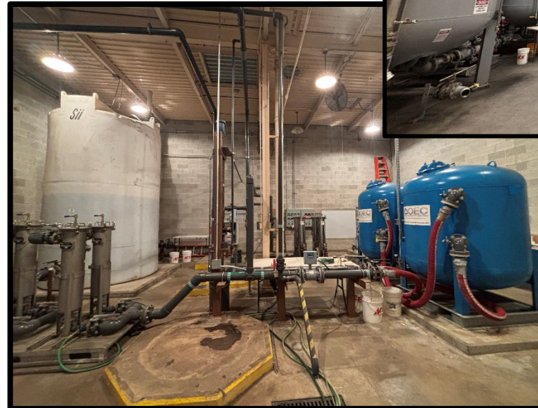
Mission Pump and Treatment System
