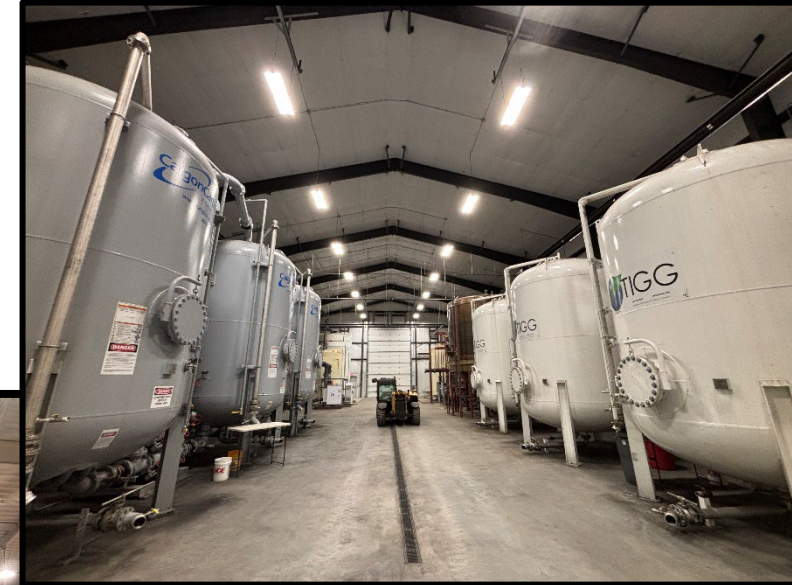
Central Treatment System 1
