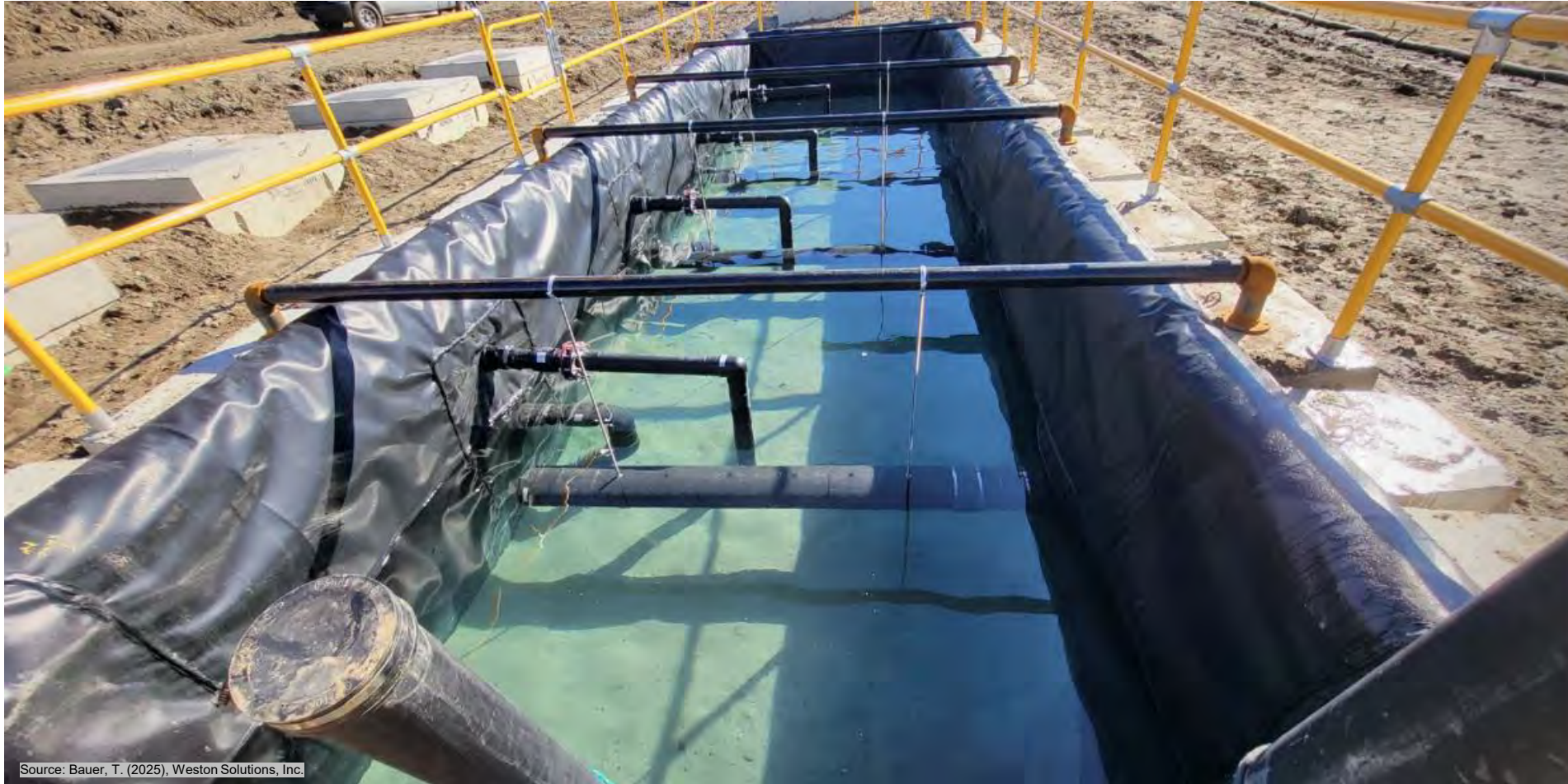
Lined gravity upflow polishing basin operating at over 150 gpm
