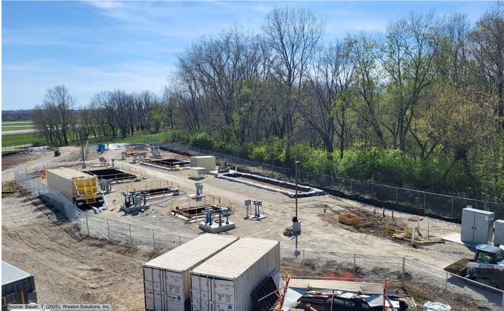
Overview of completed Area 21 Treatment System
