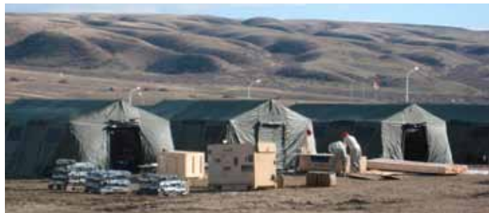
819 RHS personnel begin construction of tent flooring for the expeditionary camp at Vaziani South Training Area, Republic of Georgia
