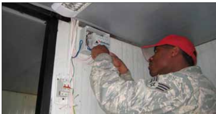
SrA Tony Rice, 819th RED HORSE Squadron Electrician, is correcting electrical deficiencies at Vaziani South Training Area, Republic of Georgia
