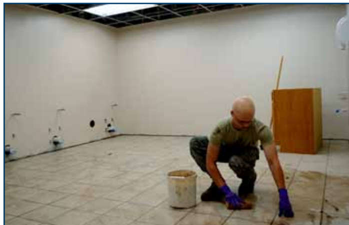
Airman 1st Class Michael Hoersten, 319th Civil Engineer Squadron, grouts tile in a newly refurbished restroom
